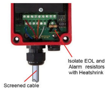
Figure 3. Control panel wiring
